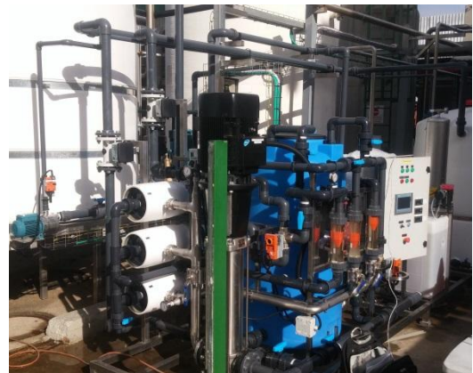
The UET unit treating the production water on site
